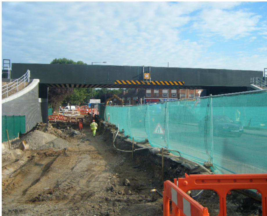
Excavation works for the new carriageways, were completed in early August near the Petts Hill Bridge.
