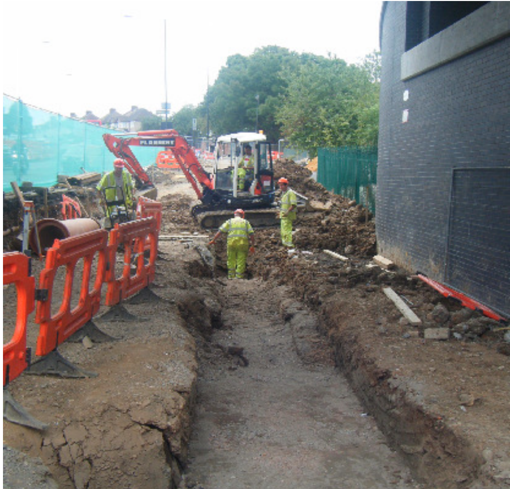
The team prepared the ground in June for future stormwater drainage works.
